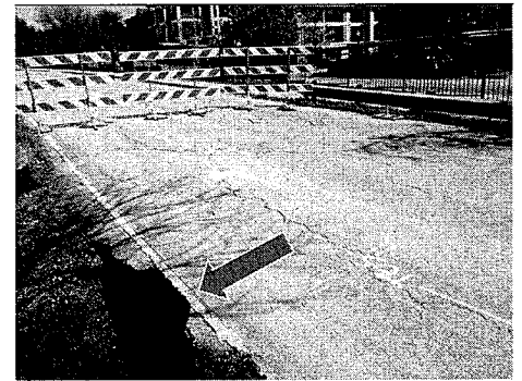
HOLE IN THE ROAD
